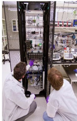
Hands-on Automation Training Automation Controllers Networks OT Software IT Software
